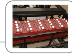
Battery: USA Trojan brand
